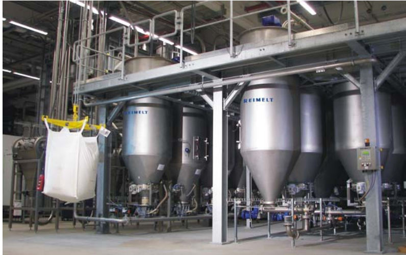
Picture 2: Receiving, storage, metering and conveying of raw materials
